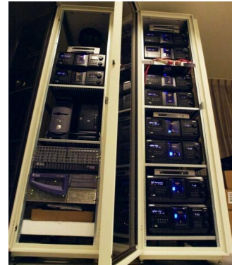
The ten CD changers, ten RBX1600s, Web server, and MP3 encoder.
